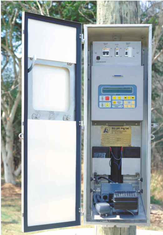
Pole Top Control & Communications Cubicle
