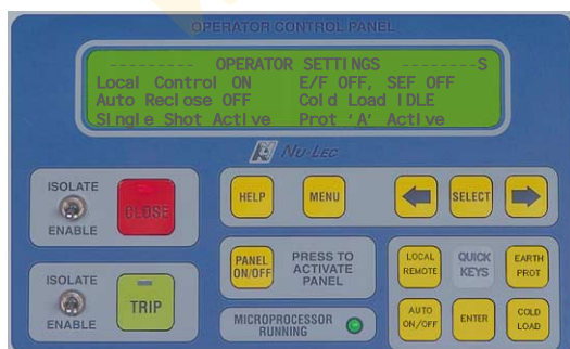
Operator control panel
