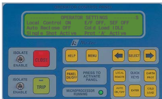
Operator Control Panel
