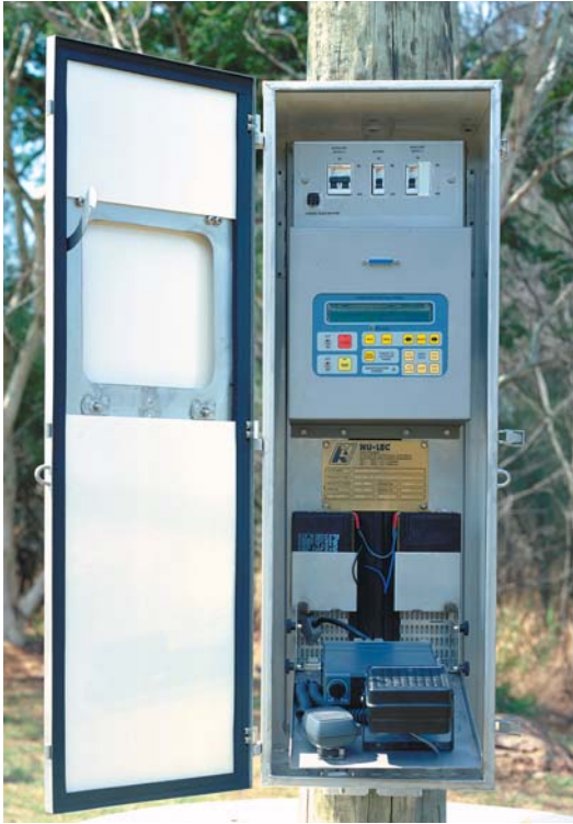
Pole Top Control & Communications Cubicle
